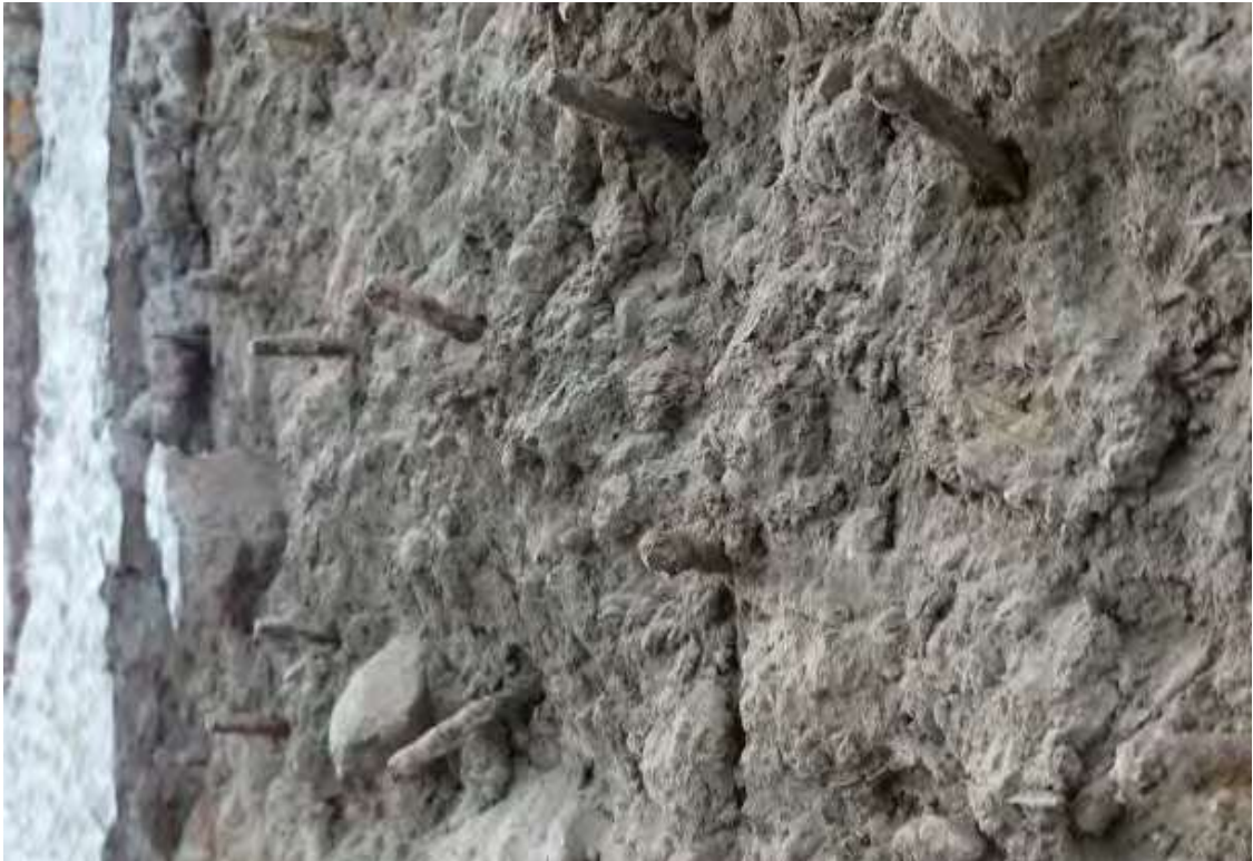
Figure 13: Some of the numerous rusted nails that had to be removed.
