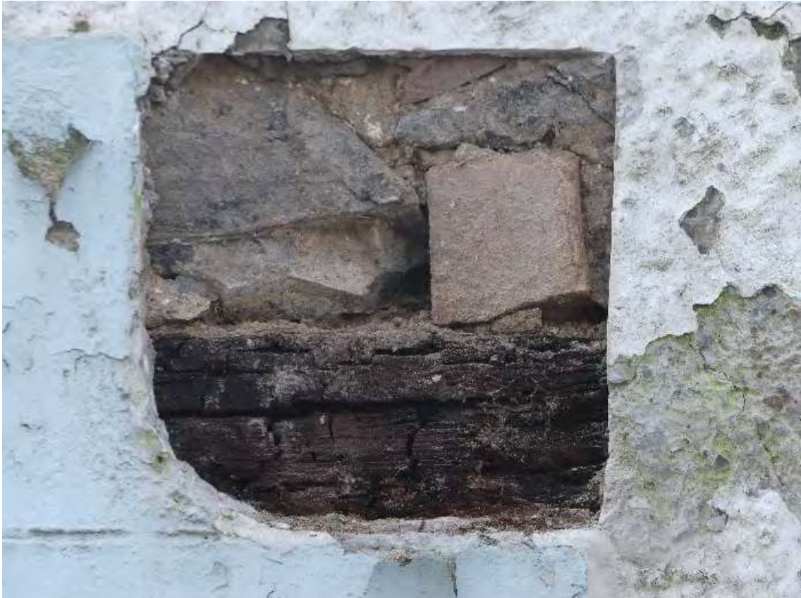
Figure 4: Inspection hole revealing a decayed timber lintel.
