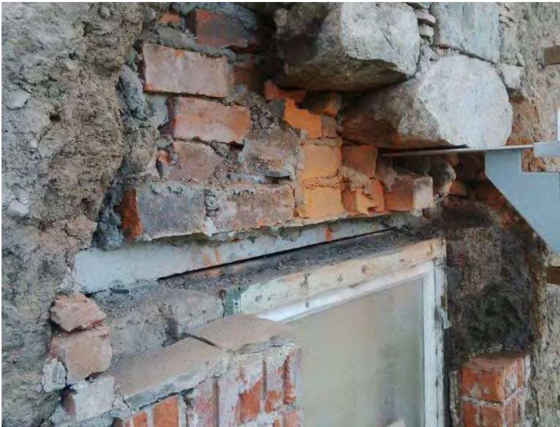
Figure 9: Temporary props allowed the lintels to be replaced in concrete and loose fill consolidated.
