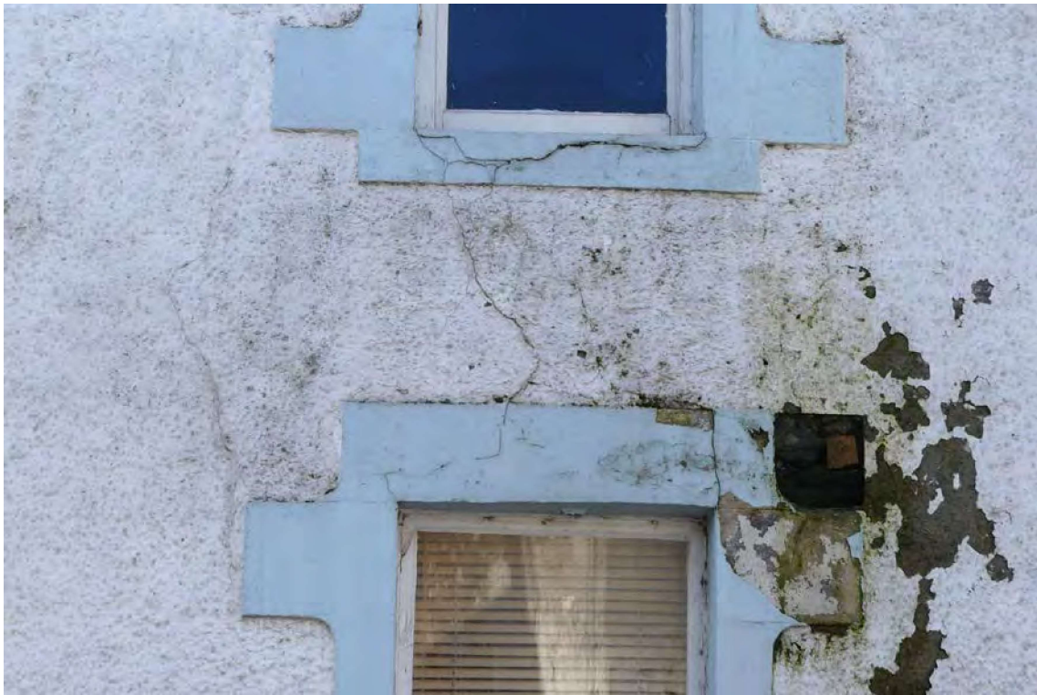
Figure 3: Cracks in the cement render
