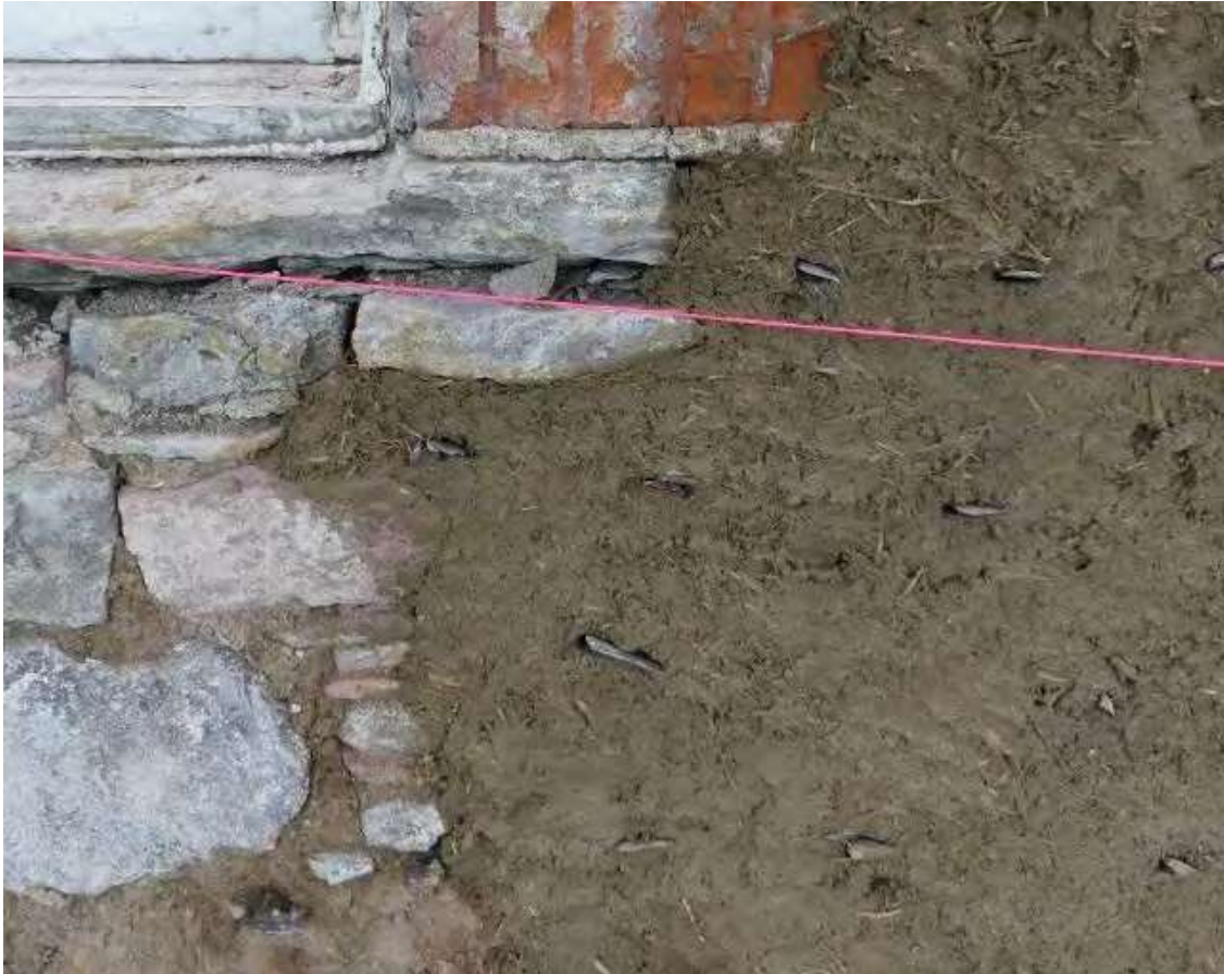
Figure 15: Slate hammered into the daub, with strings used to set a face line.
