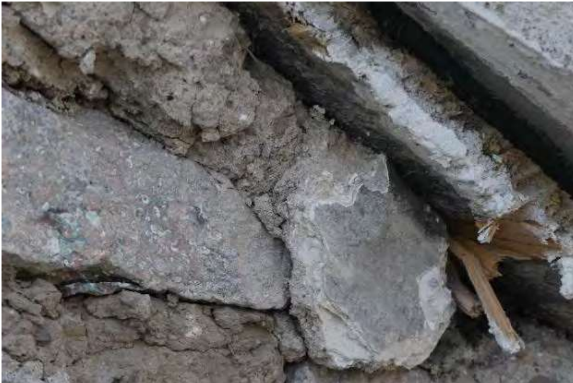
Figure 18: One fragment of original lime harl with limewash was found beneath the cement render.
